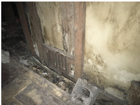
Mold growth in the boiler room area
