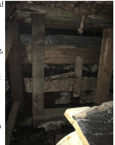
Deterioration of skirting & posts
