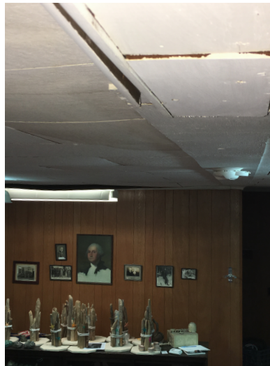
Sag in Meeting Room ceiling
