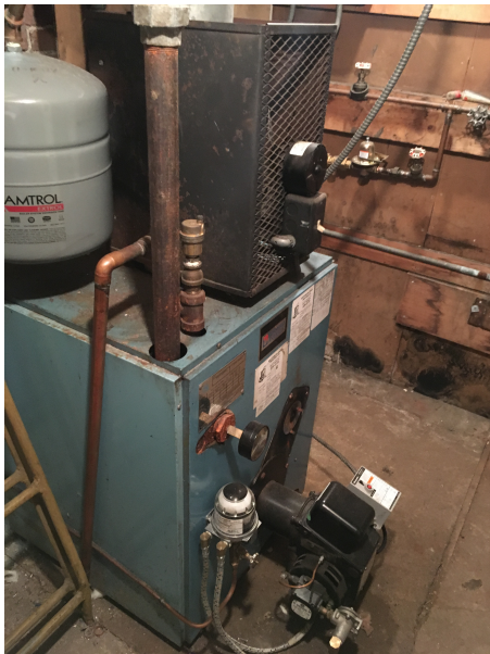
Existing boiler in crawl space
