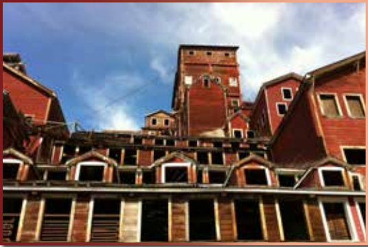
Mill building, Kennecott Mines NHL, Wrangell-St. Elias National Park and Preserve. (OHA photo)
